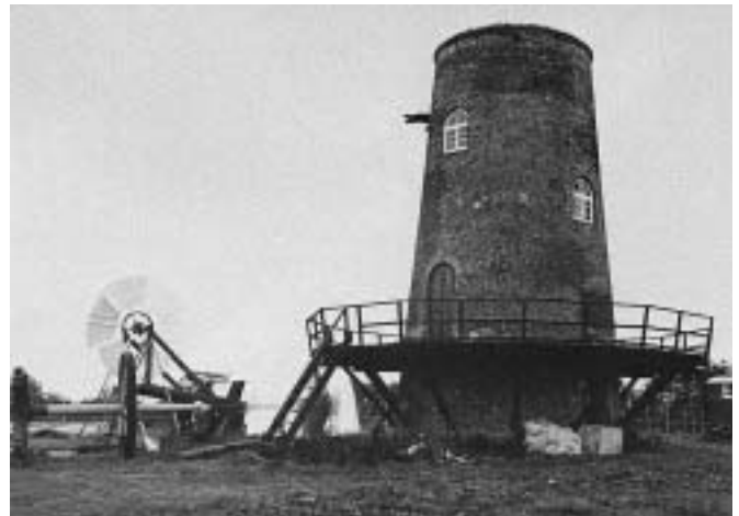
Works underway in 1975. The tower has been restored, the gallery constructed and the fantail is being assembled.
